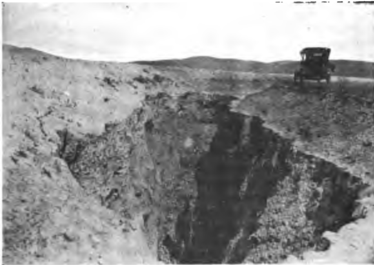
FIG. 72.—Cavity Developed in Canal Bed, Flathead Reservation, Montana.
